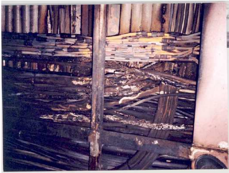
Photo 2. View of burned cabling above deck of engine control room (note effect of heat on copper tubing)
