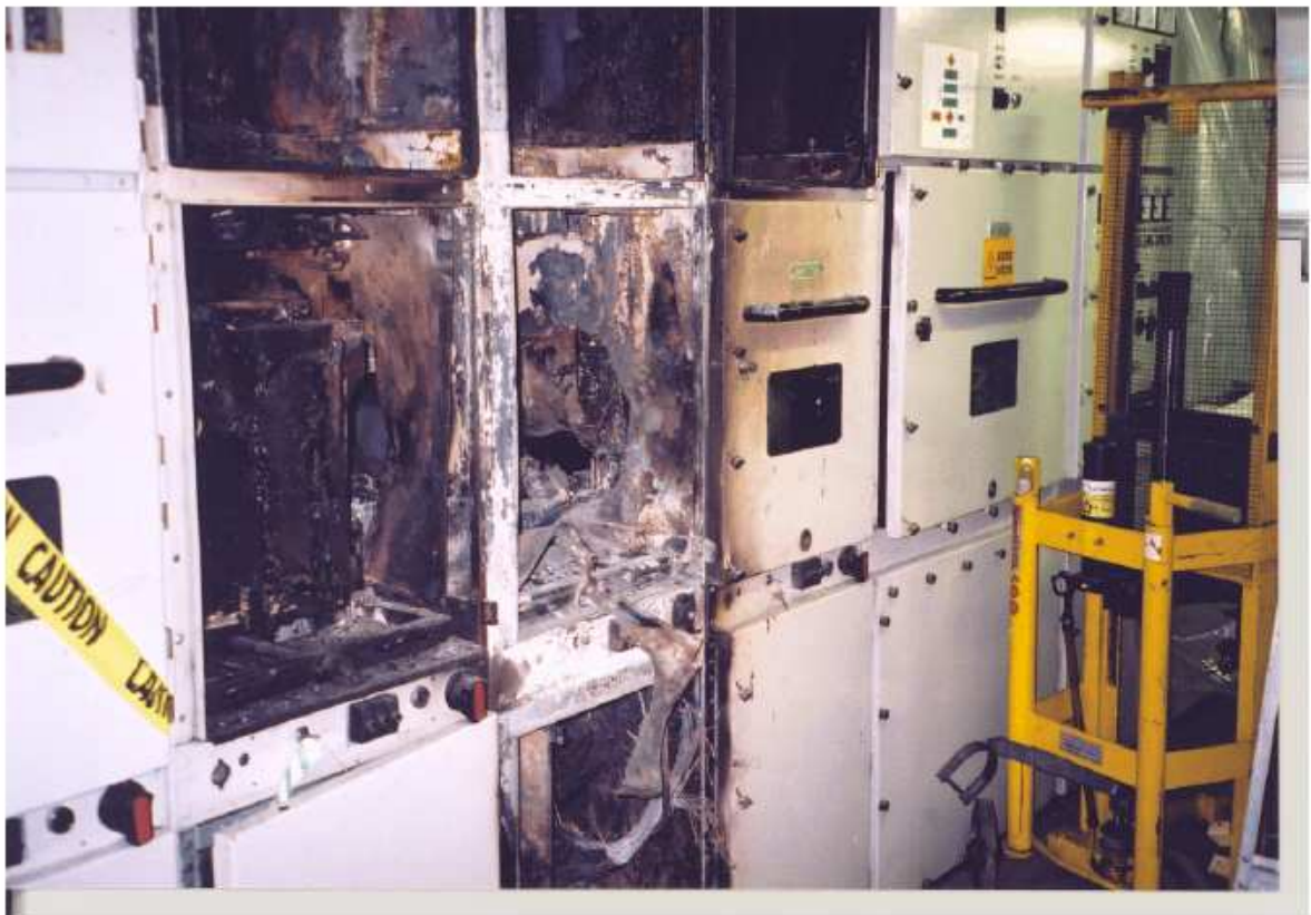
Photo 1. View of DG 2 circuit breaker and relay consoles. DG 1 and bus-tie breaker consoles are on either side.
