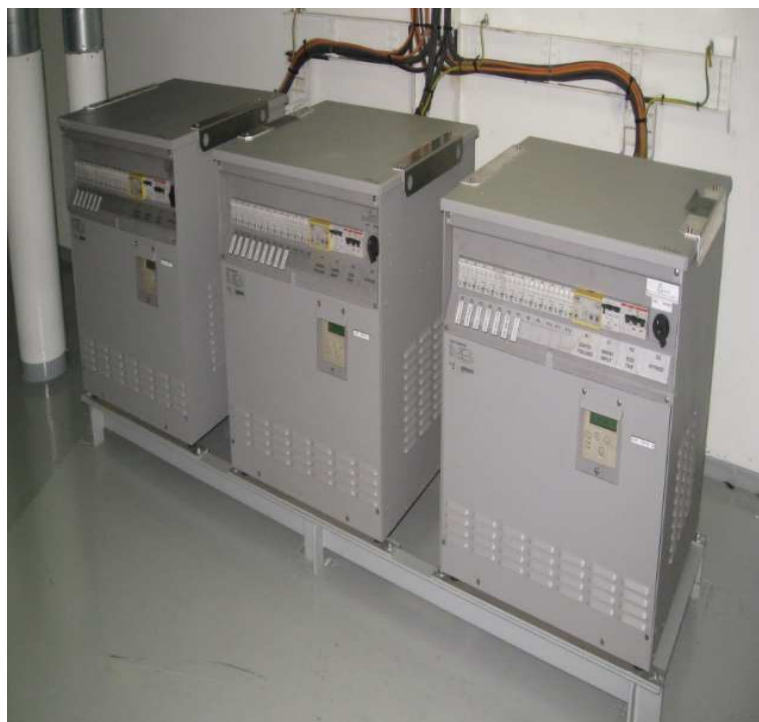
(Figura 7 – Uninterruptable Power Supply- UPS)
